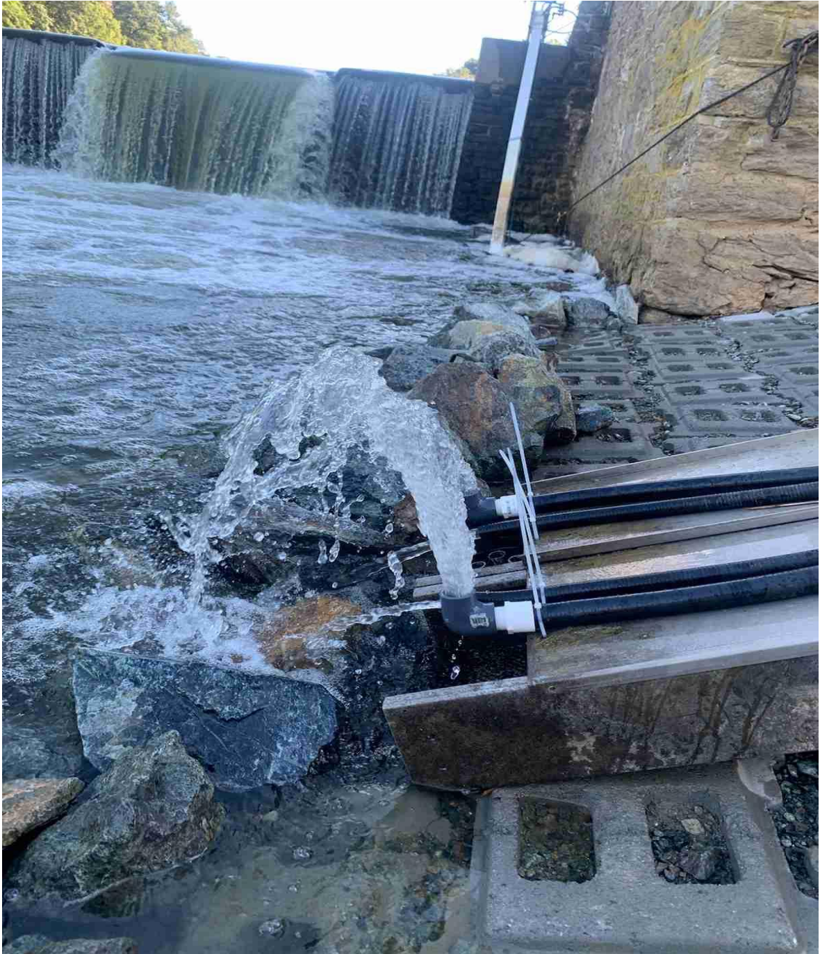
Figure 3.1-2: Ramp Entrance during 2022 and 2023 Eel Collection Seasons at 182 cfs, Octoraro Creek Eel Facility, 2024
