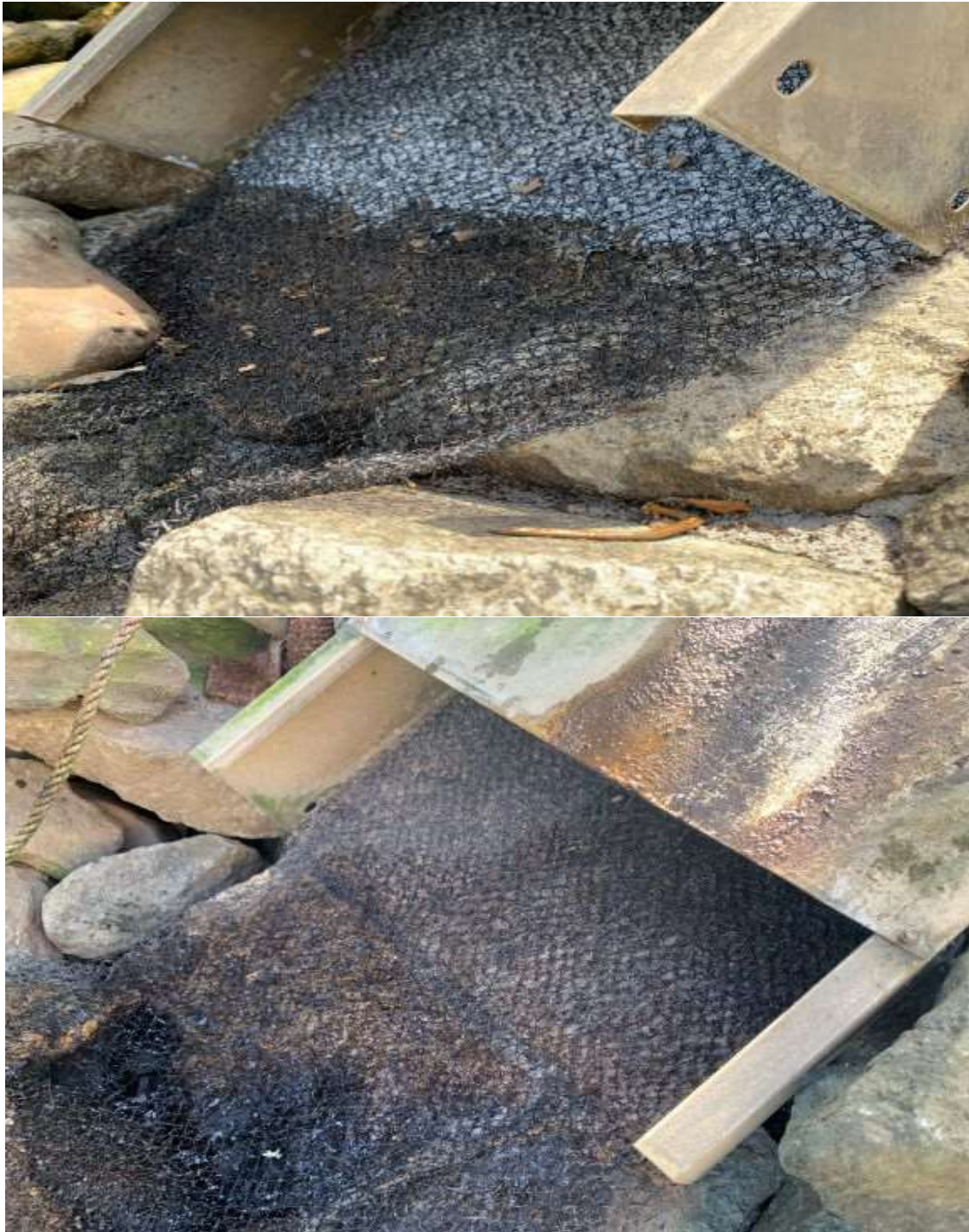
Figure 5.0-1: Transition from Riprap Shoreline to Ramp Entrance, Conowingo West Eel Collection Facility, 2023
