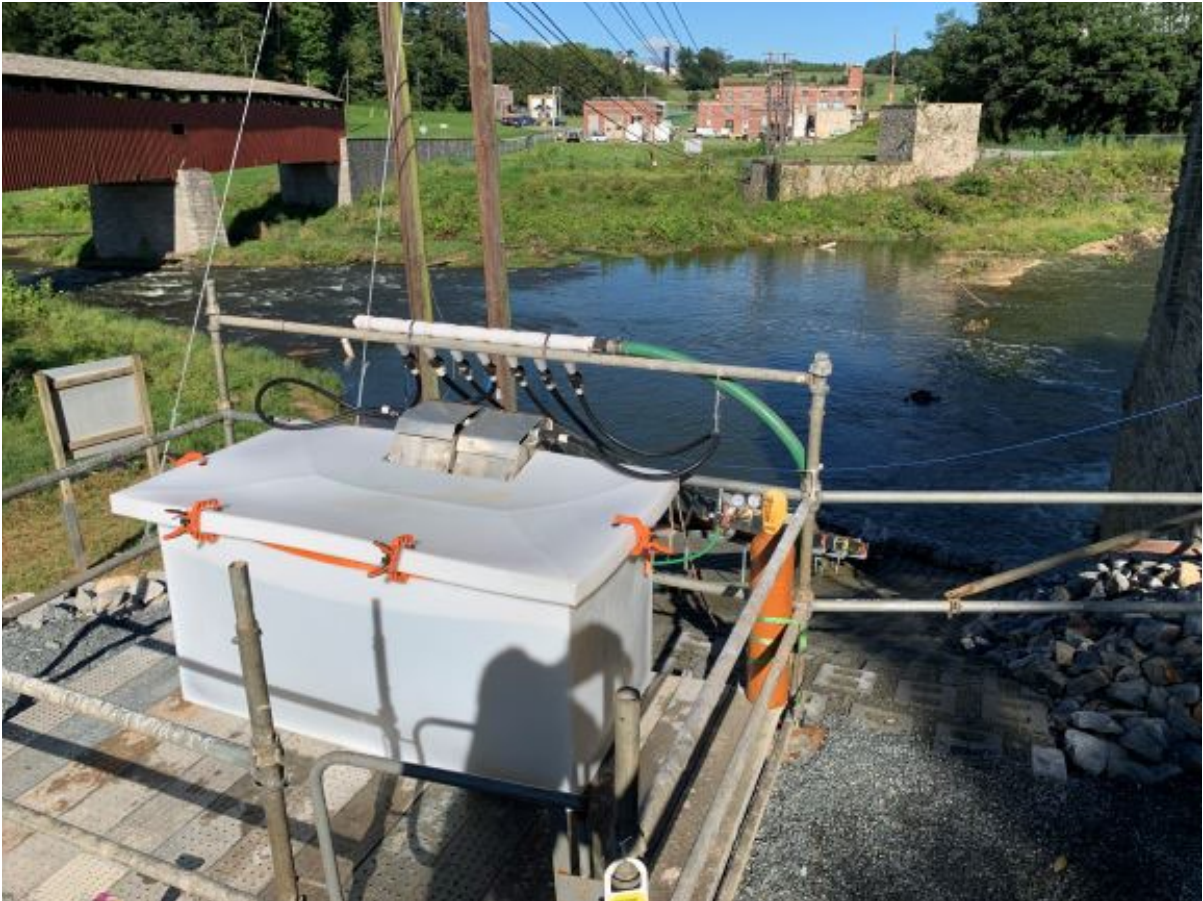
Figure 3.1-1: Scaffolding and Collection Tank on top of the hill, Octoraro Creek Eel Facility, 2022
