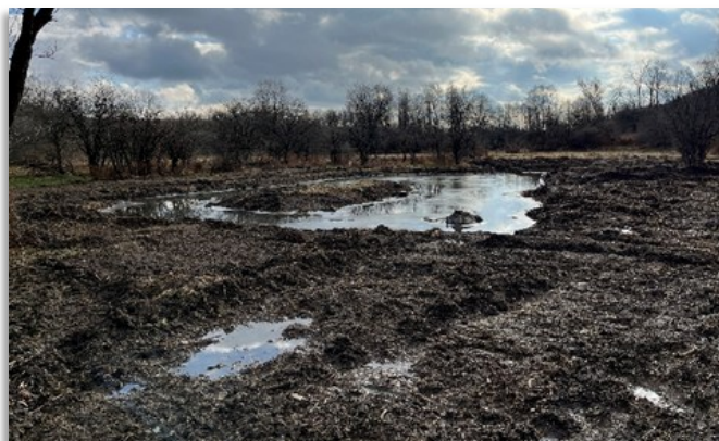
Potholes under construction
